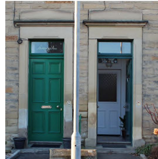
Figure 29: Matching Traditional External Doors (with internal door in entrance) - retaining matching doors on a street assists in protecting the character and appearance of the street.
