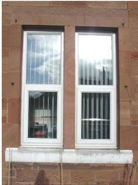
Figure 20: Replacement Window within stone opening, with mid hung sash. This results in a 'heavy' appearance on the lower half of the window.
